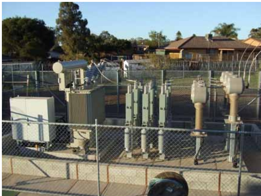
Figure 3.3: Ripple Injection Equipment at a Zone Substation (photograph courtesy of Essential Energy)
